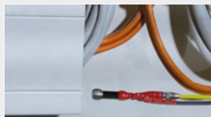
Shafts and underfloor ducting
